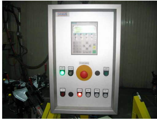
Fig. 23: Green button on the control panel, indicating that all parts are well fixed and the welding process can begin [own study].
